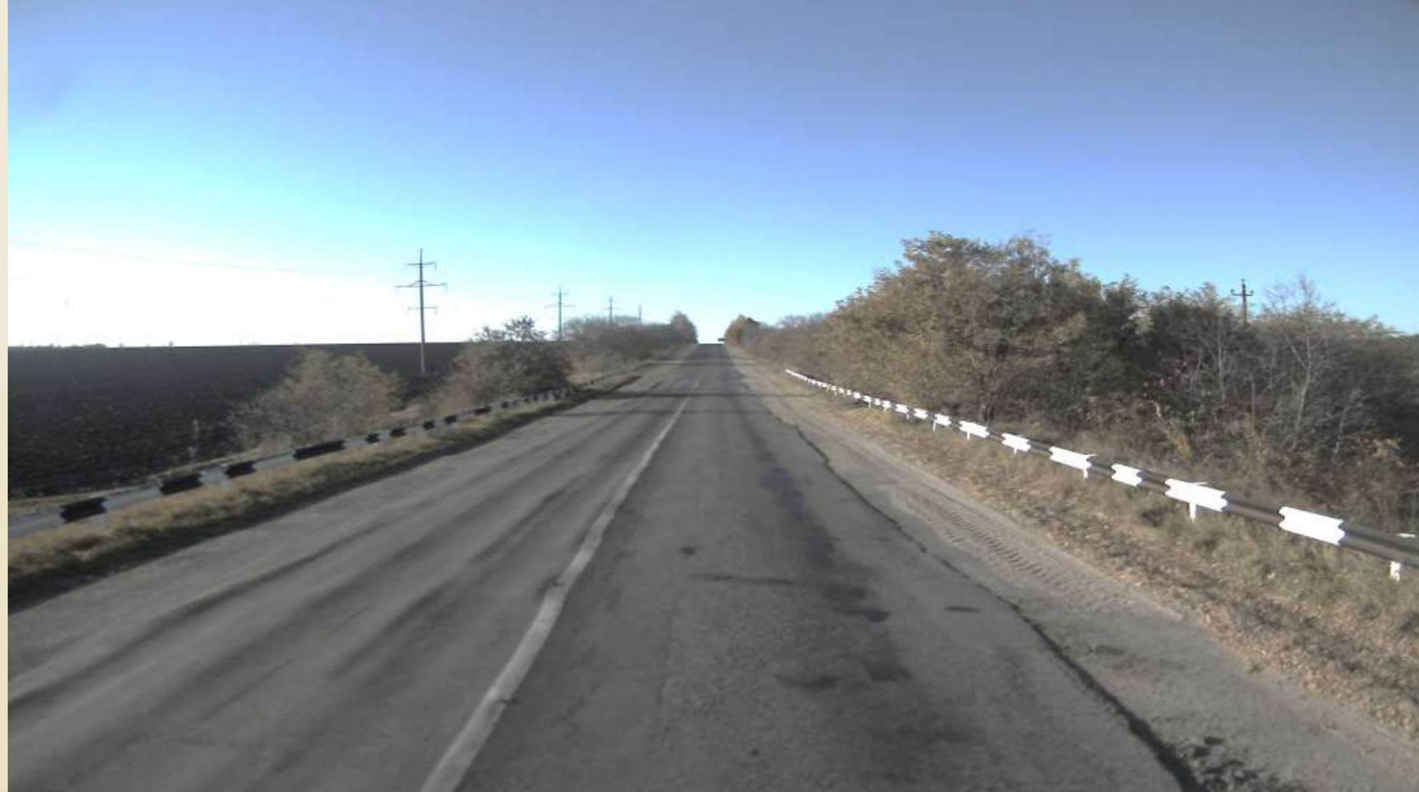
R7 - (PCI - 4 - Destroyed)
